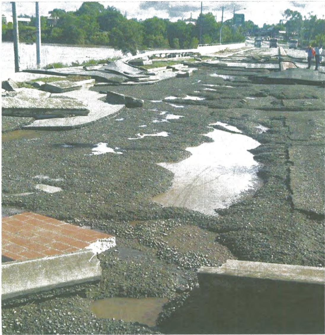
MAJOR PROJECT: The damage at the One Mile bridge caused during flooding earlier this year.
